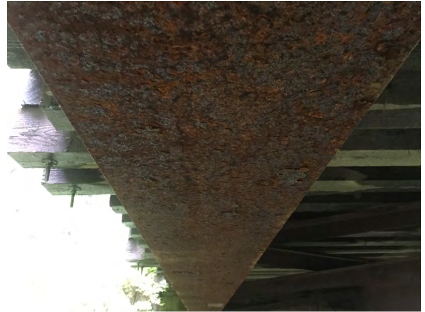
Slight corrosion noted on superstructure
