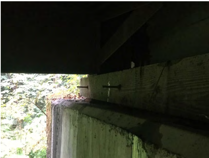
Right bank, downstream girder shimmed at bearing
