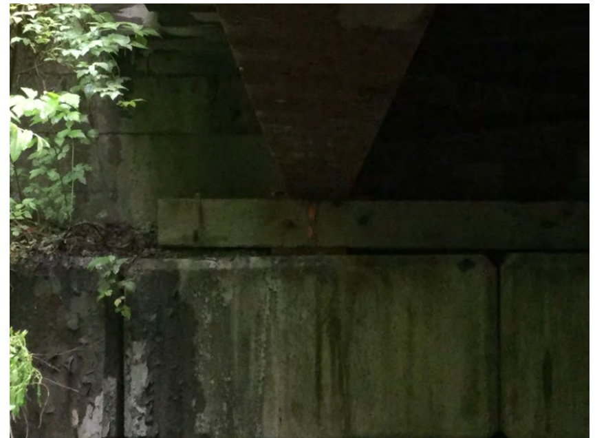
Left bank, upstream girder shimmed at bearing
